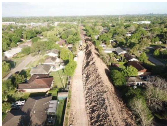
Aerial photo of the work being done between Sanford and Kingfisher for the new culvert to the Willow Waterhole basins.
